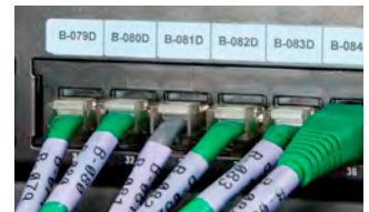
Patch Panel Labels
