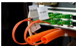
Fiber Optic Cable Markers
