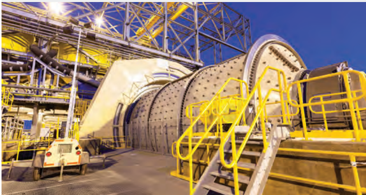
③ Power Quality & Power Distribution
